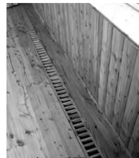
Outlet of underfloor heating
