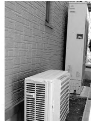
High-efficiency water heater
