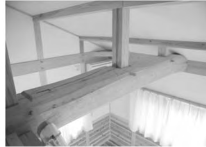
Beam made of recycled timber
