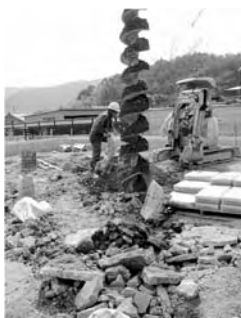
Pillar-shaped improvement pile
