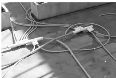
Water supply header
