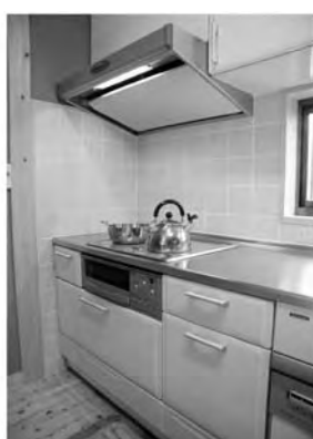
Induction-heater (IH) stoves
