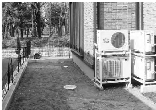
Site of the air conditioner outdoor unit
